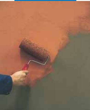
Example of an application of Elastocolor Rasante with a porous sponge roller
