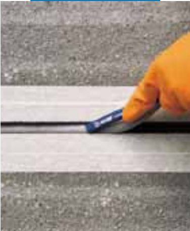
Protection of the joint edges with a protective tape and positioning Mapefoam into the joint
