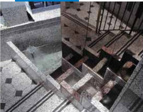
An example of an installation of a granite floor and wall with Keraquick + Latex Plus - Caesaris Palace in Merseyside - Liverpool (GB)
