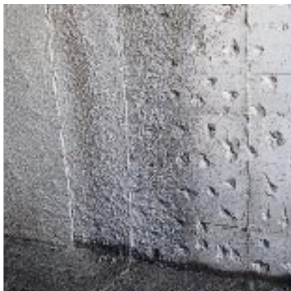
Applying mortar admixed with IDROSILEX over concrete roughened with a bush hammer
